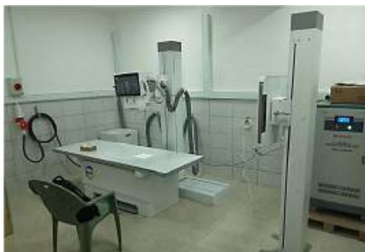
X ray machine installed at SDA Better Living Hospital.
